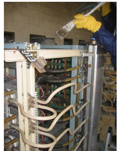
Dry Ice Cleaning of Thyristor
