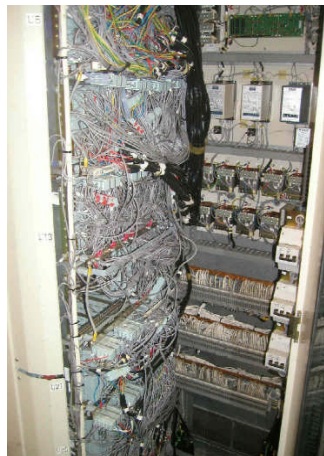
Electrical Switch Cabinet opened for detail cleaning
