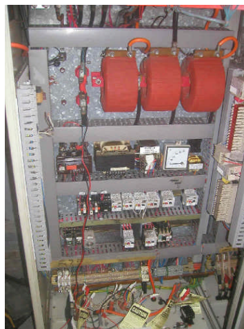
Electrical cupboard opened during cleaning process
