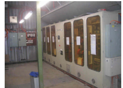
Switch Room fully decontaminated
