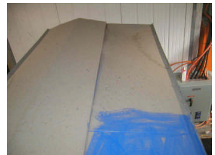
Contamination on top of electrical cupboards before cleaning
